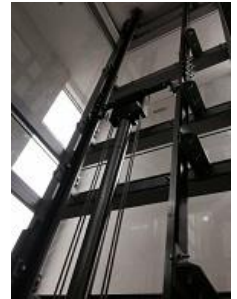
CUSTOM PAINTED MECHANICAL
